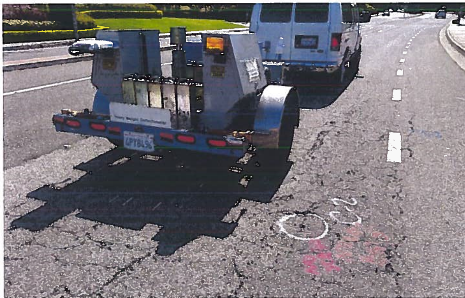
Photo 6: Pavement deflection testing being performed at coring location C-2 within an area of medium-severity alligator cracking on Ford Road, Newport Beach.
