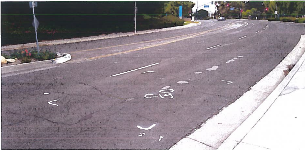
Photo 5: Coring location C-19 on Enterprise in Aliso Viejo. Pavement contains alligator cracking, depression, and potholes.
