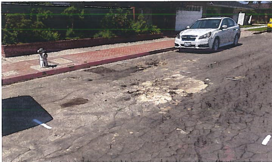
Photo 7: Condition of the pavement within Cameo Highlands, Newport Beach, prior to improvement.
