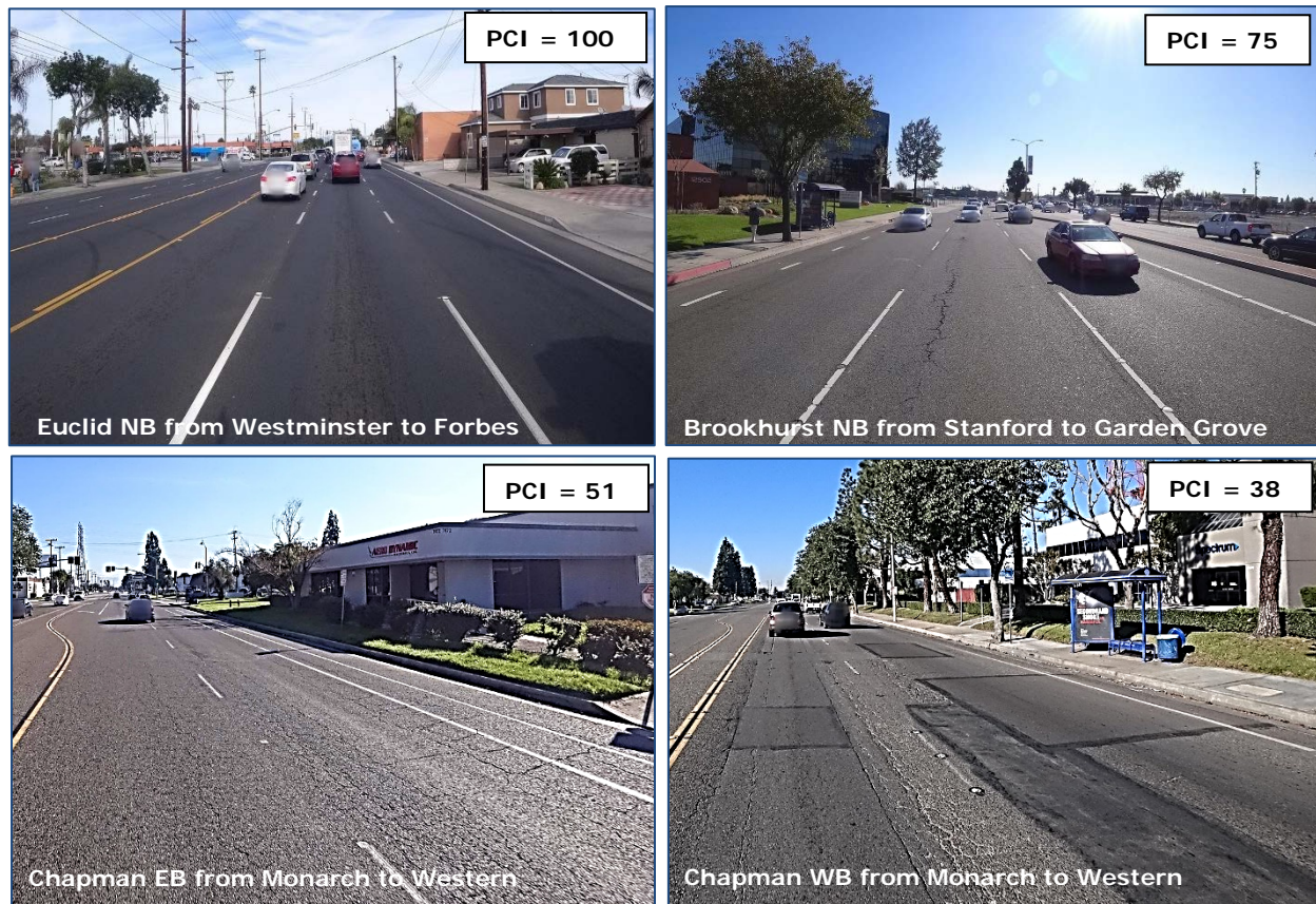
Figure 1: Pavements with Various PCI's
