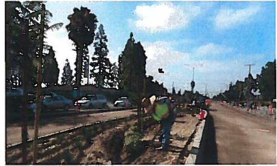
Euclid Street/Garden Grove Blvd/Woodbury Avenue Rehabilitations and Palmwood Sidewalk, City of Garden Grove
