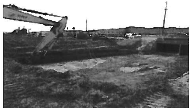
Line D and Line D-1 Storm Drain Realignment Project, City of Murrieta
