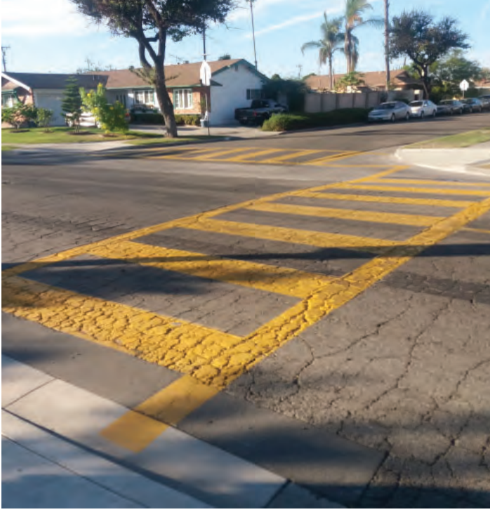
High visibility crosswalk on top of cracked pavement.
