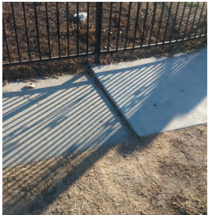
Uneven sidewalk on Woodbury Ave.
