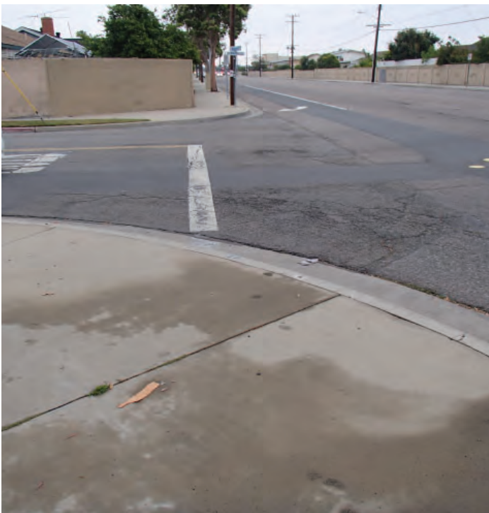
Missing ADA compliant curb ramps along Hazard Avenue at Kerry Street.
