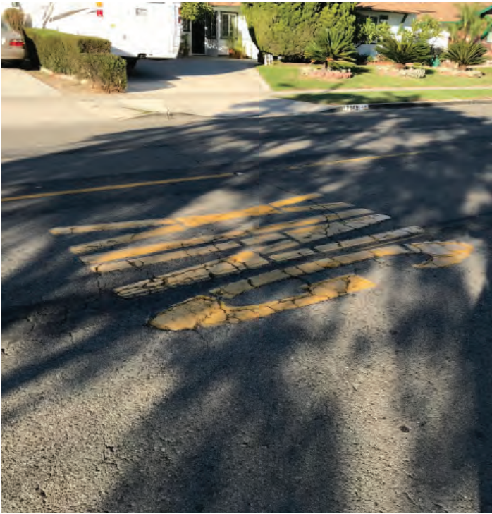
Fading school pavement markings on Woodbury Avenue.
