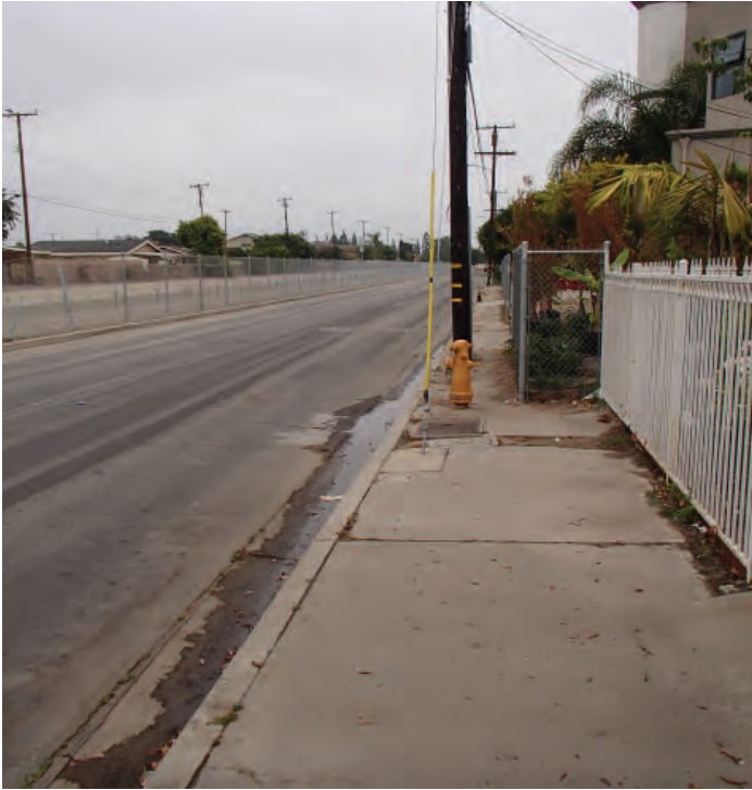
Incomplete sidewalk along 13th Street. Sidewalk ends at the fire hydrant followed by dirt path.
