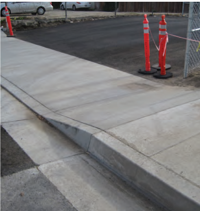
Recent sidewalk improvements at staff parking lot driveway along Bushard Street; not ADA compliant.
