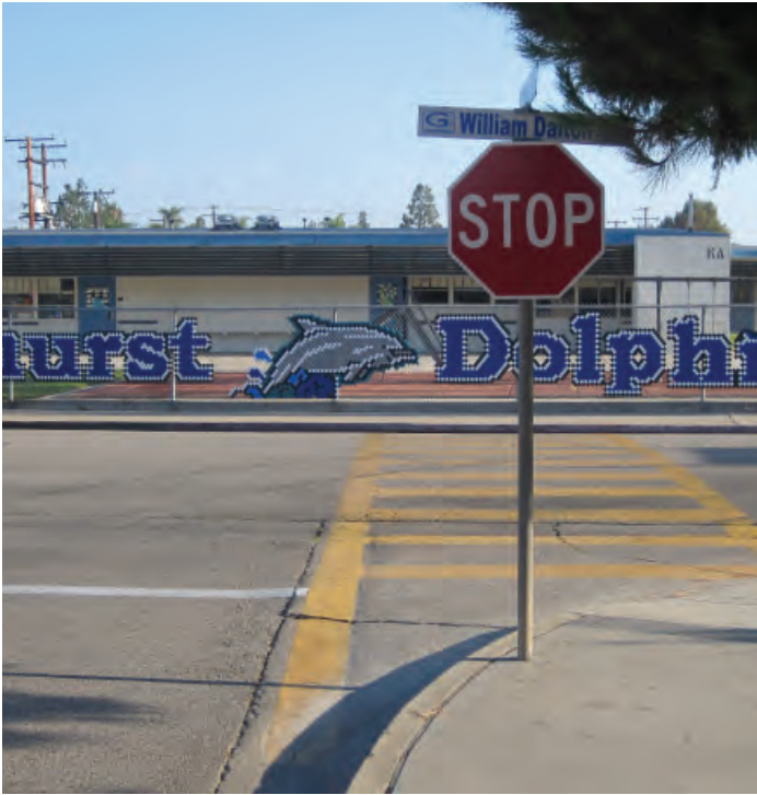
Faded crosswalk & missing curb ramp on William Dalton Way and Hester Place .
