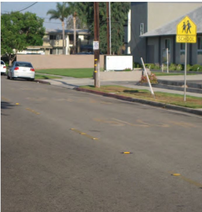
Faded school pavement markings on Bixby Avenue.
