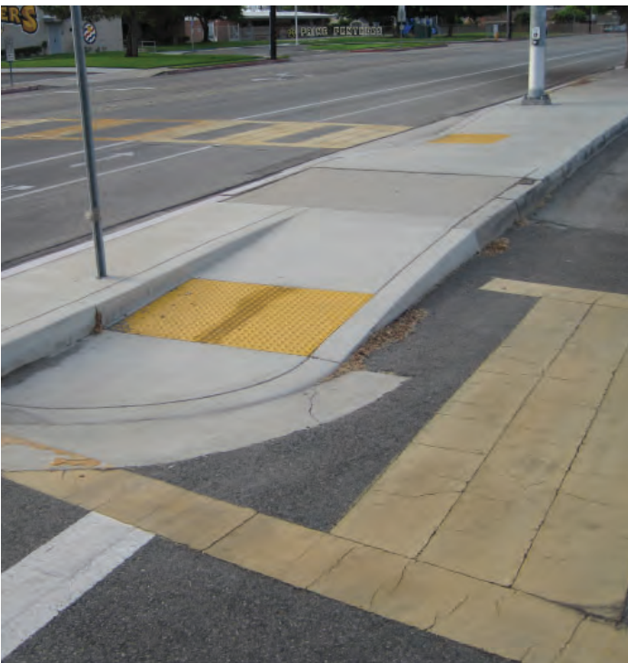
ADA compliant curb ramps provided at existing pedestrian signal crossing and adjacent roadway.
