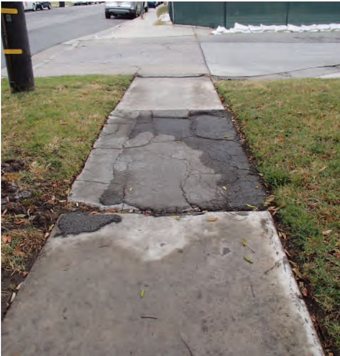
Sidewalk improvements needed along 11th Street to eliminate tripping hazards.
