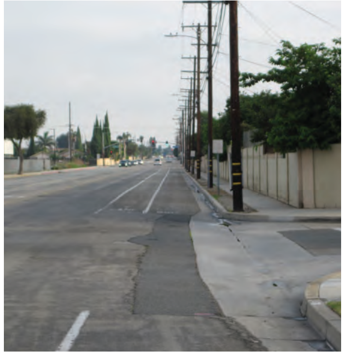
Bike lanes with faded pavement markings and missing signs.
