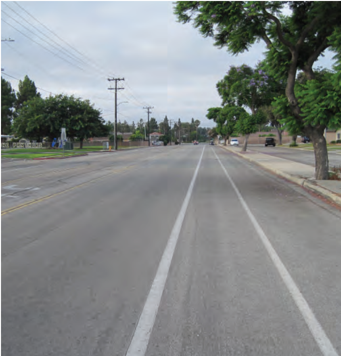
Faded roadway pavement markings along Ward Street.
