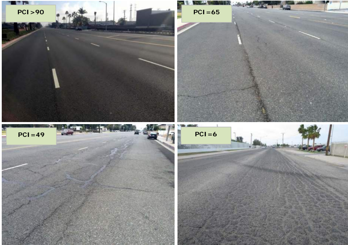
Figure 1: Photos of Pavements with Different PCIs
